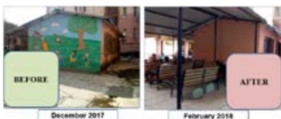
Waiting area constructed for DR-TB patients with open shed and improved ventilation, Urban Health Center, Dharavi, Mumbai, India.
