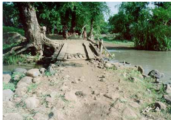
A bridge on the verge of collapsing
